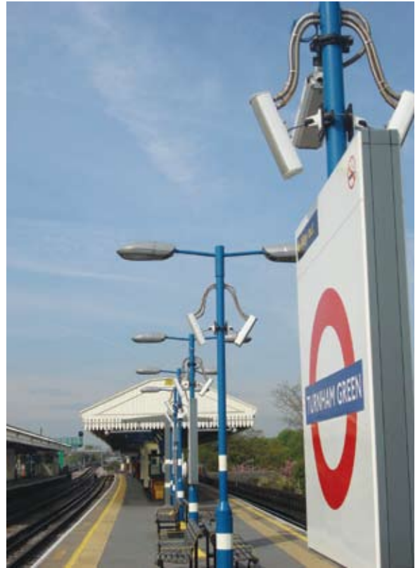
Typical station public address relies on large numbers of speakers to flood the platforms with sound, which can result in noise pollution and poor audibility.
